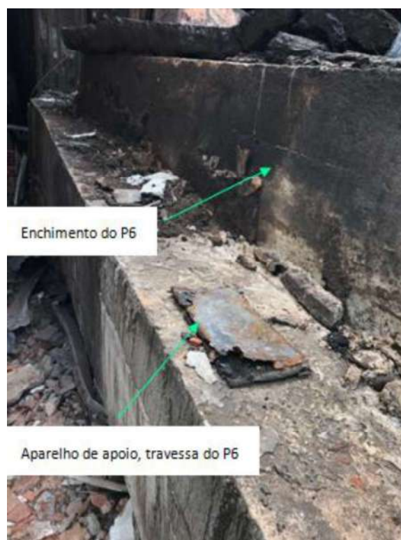
Figure 7 - Cap beam, bent P6, where it can be identified the slab bearing device, source: Authors
