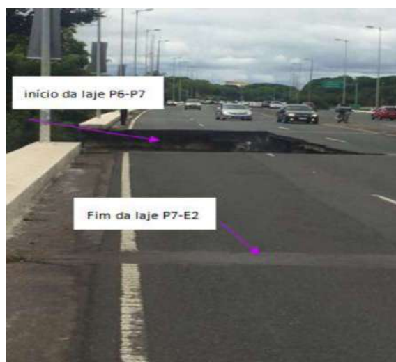
Figure 5 - Partial collapse of the deck, Source: public
