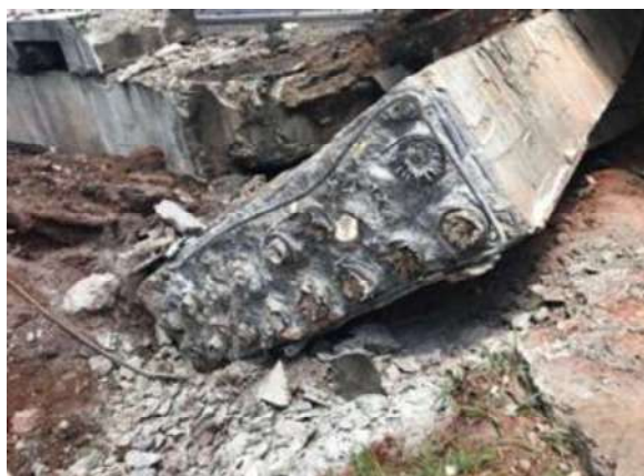
Figure 9 - Detail of the cable anchors in the end section of the cap beam, P7, with 16 cables, with 18 wires of 5 mm in each, Source: Authors
