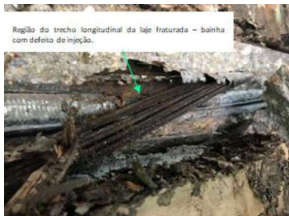
Figure 8 - P6-P7 span sheaths photo, where it can be identified sheath without injection, Source: Authors
