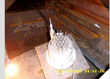
Load cell on the anchorage
